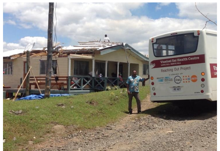
Badly damaged Nurses Quarters at Waimaro Nursing Station
